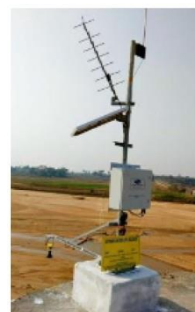
Flood Monitoring Station
