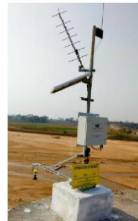
Flood Monitoring Station
