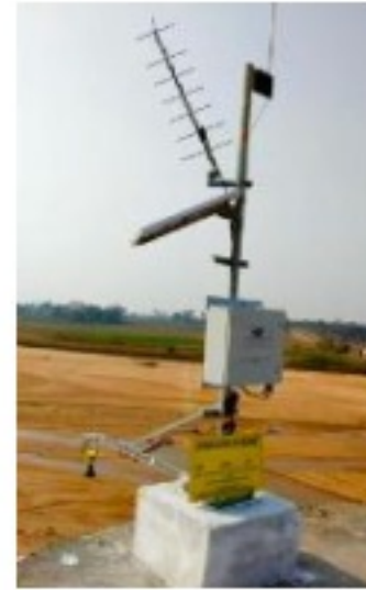
Flood Monitoring Station
