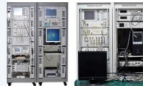
ATE ATS - Facility
